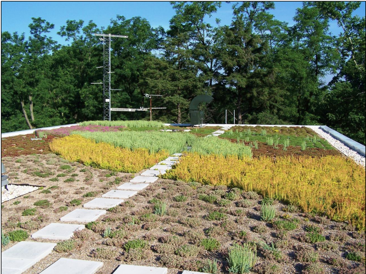
A green roof on the Media Production Center improves insulation, minimizes stormwater runoff, and reduces the heat-island effect.
