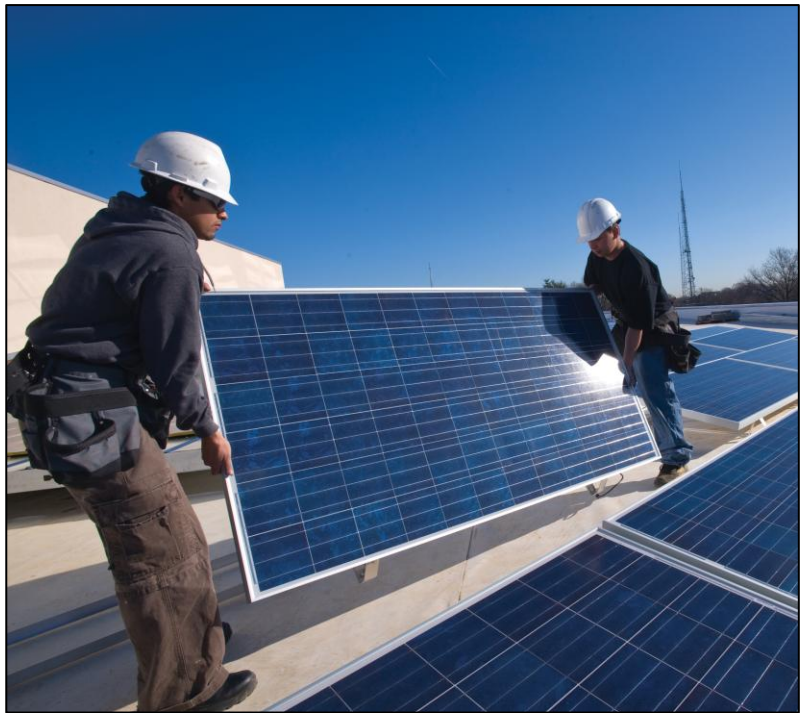
The new School of International Service features a 33kW rooftop solar photovoltaic installation.
